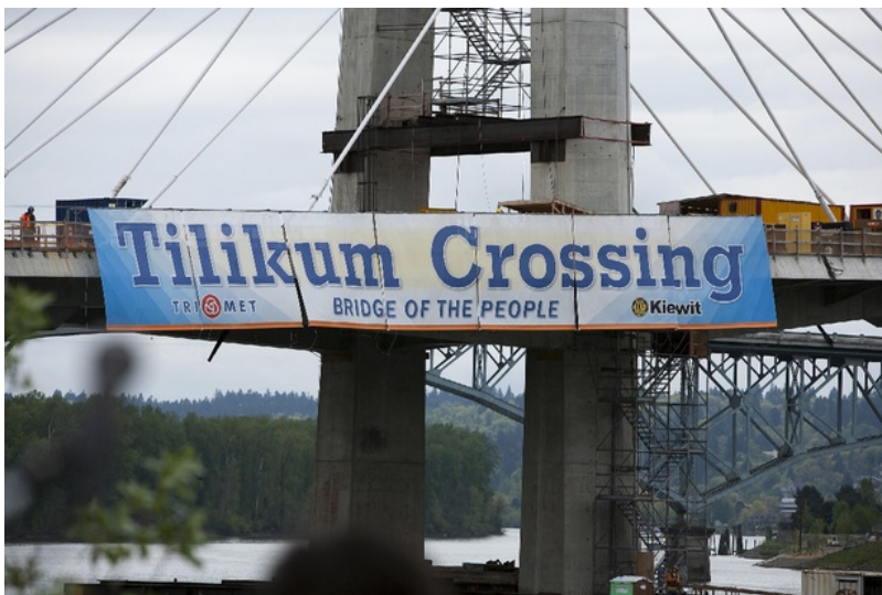
Tilikum Crossing (top, April 2014 construction) is expected to open in fall of 2015. ( TriMet / Flickr )
