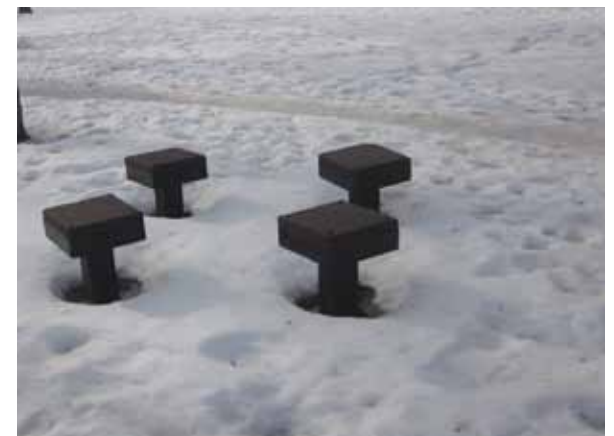
The state of existing infrastructure exemplifies the need for improvements in management and maintenance, as well as capital investments.
